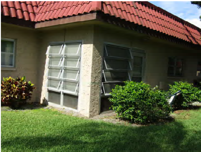
No window or door protection
